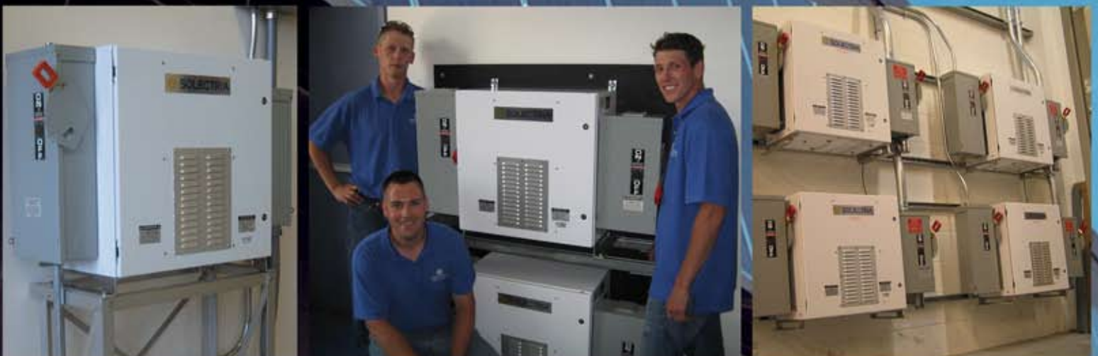
Background & Left: 13.8 kW system at Evergreen Solar's mfg. facility Center: 35 kW NexAmp installation at Ebsco Publishing Right: 120 kW system (4 of 8 inverters) by Chico Elec/Solar Design Assoc, AT&T Park, Giant's baseball stadium, San Fran, CA
